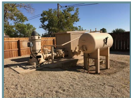
California City water infrastructure
