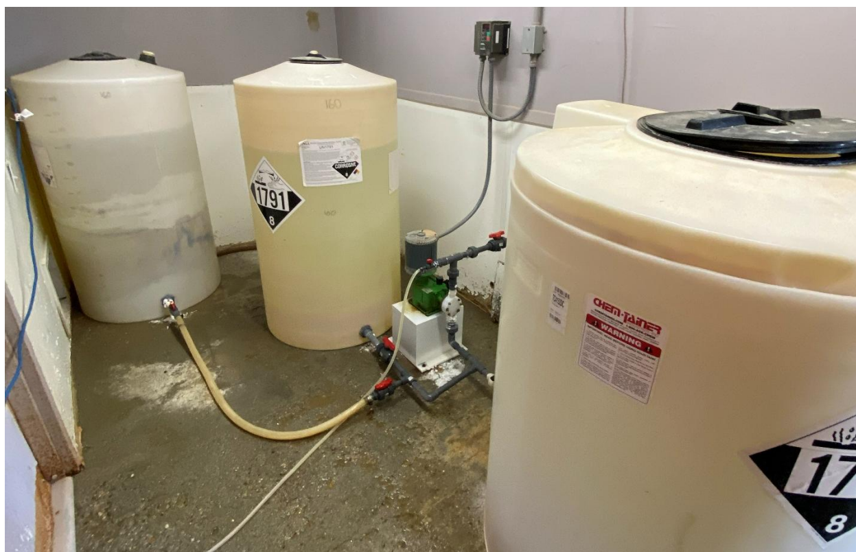
Figure 5-2 Well 14 Chemical Injection
