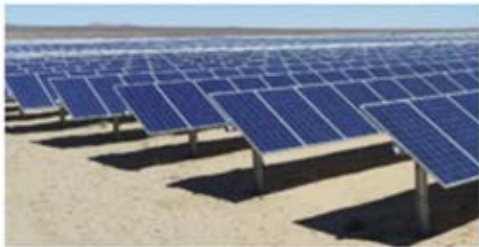
Typical Single-Axis Tracking Solar Panels
